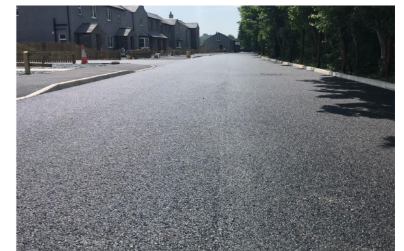
Asphalt surfacing to northern arm of Wolfe Tone Square and Teeling Street
