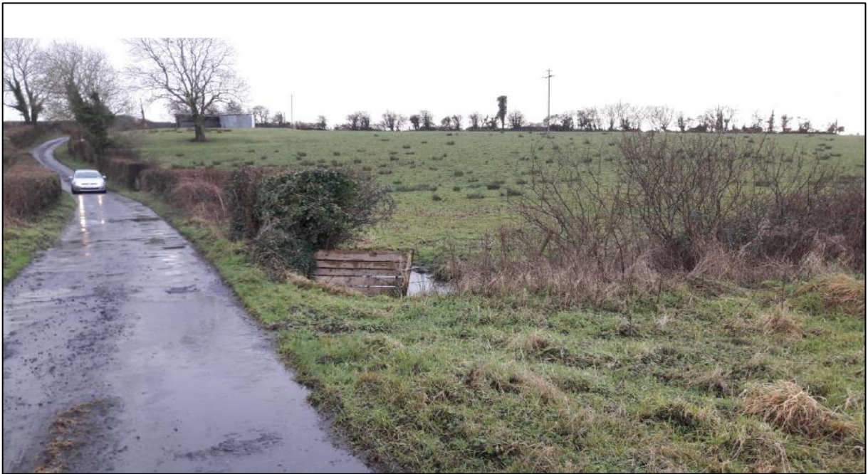
Figure 2.3a View of site from Robber's Lane looking South – pallet marks culvert for stream under road.
