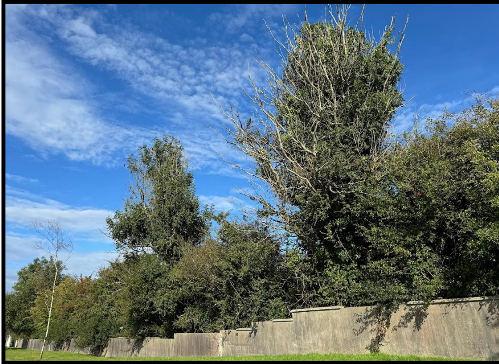
Image of the southern boundary looking west along River Walk. Tag 368 & T369 in view.
